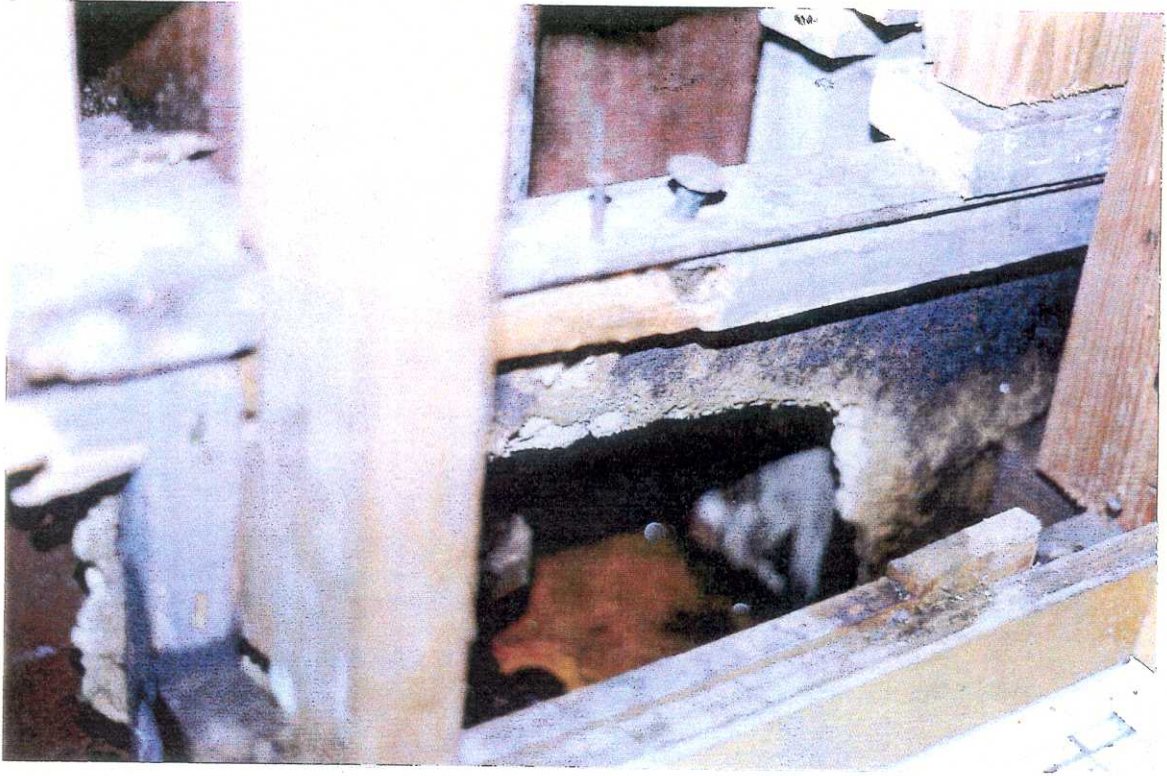
TYPICAL ASBESTOS INSULATION INSIDE WOOD PANELING
