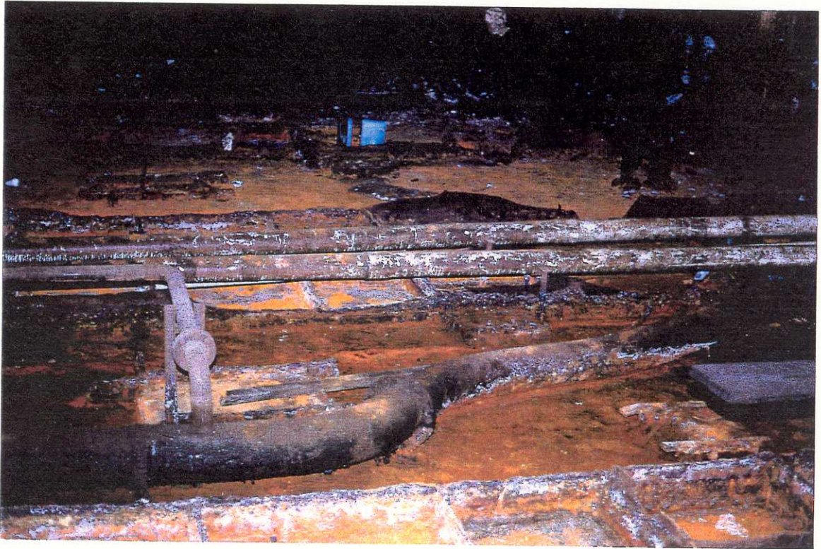
FWD TURBO GENERATOR ROOM - BILGE
